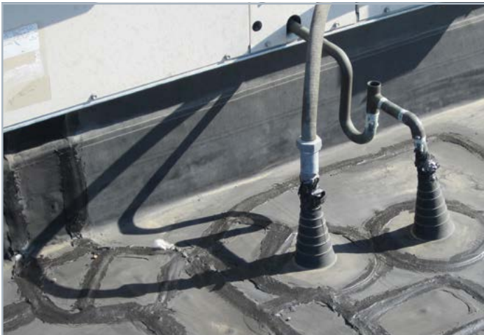
1. Address all problem areas. Repair with like materials. Clean the roof, removing dirt and debris.
